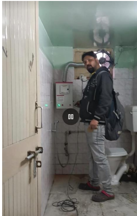
INCINERATOR IN STAFF TOILET
