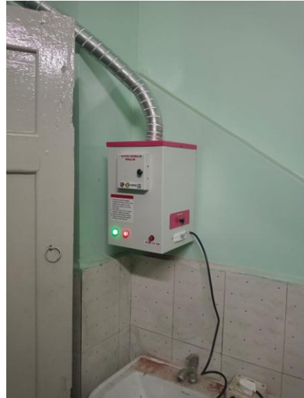
INCINERATOR IN GIRLS' WASHROOM
